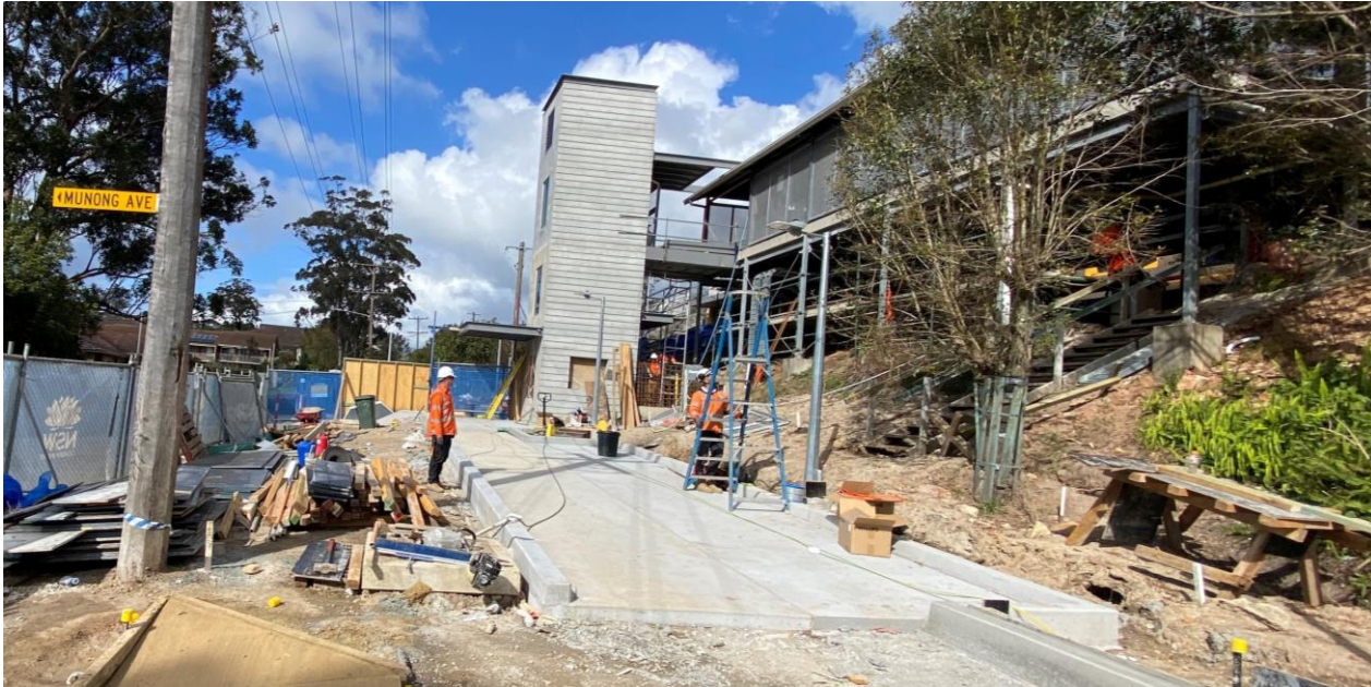
New station entry on Kurrawa Avenue with concrete works progressing and lift fit out underway
