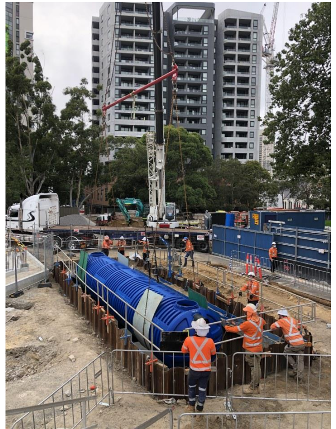
Above: the water tank in place within the Marian Street compound and almost ready to harvest rainwater.
