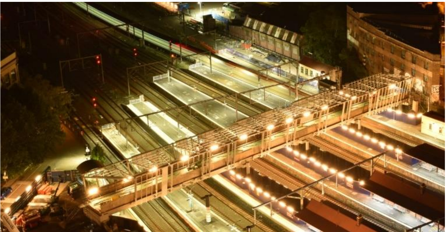
Photo: the final installation of the bridge canopy structure at Redfern Station in December 2021.
