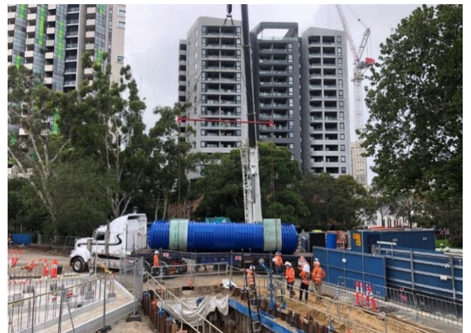
Above: the delivery of the water tank into the Marian Street compound and the crane in the background about to lift it into place.
