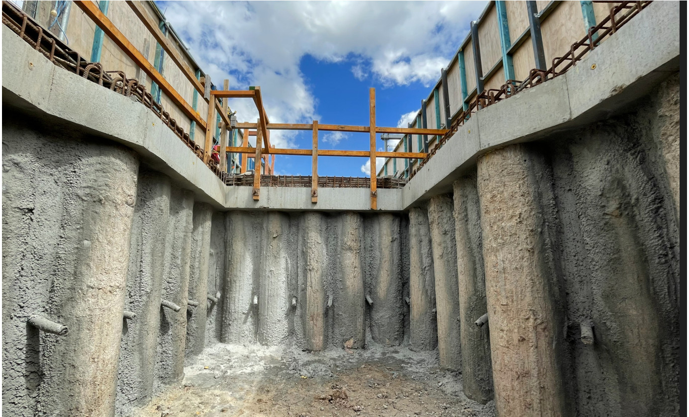
Pictured: The platform excavation in November, where the lift will eventually be located.
