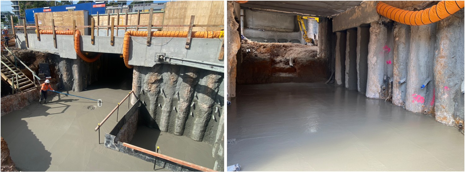
Left image: Concrete placed in the new Waitara Avenue Car Park underpass entry and lift pit. Right image: The newly excavated underpass from the car park to the island platform completed during December.
