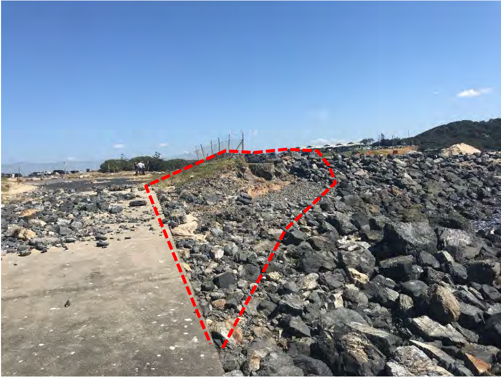
Figure 24: Damaged area – ramp shows “wash-over” material from eastern side of ramp, indicates damage also occurring on eastern side of ramp
