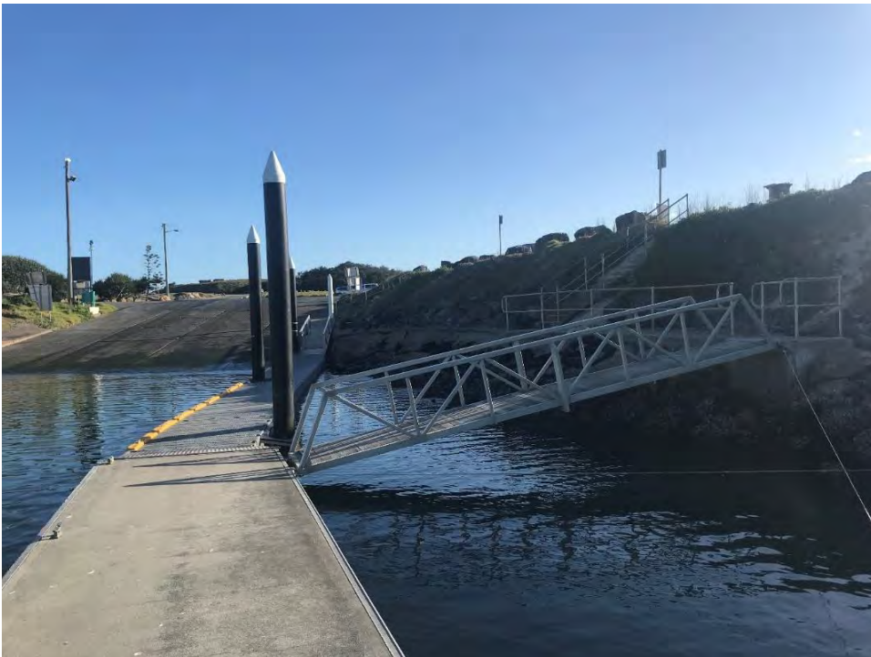
Figure 19: Existing Pontoon – minor repair works required
