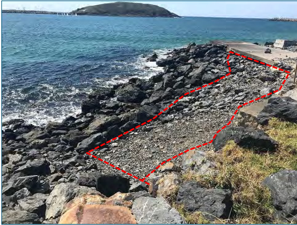
Figure 21: Damaged area west of existing Material Offloading Ramp
