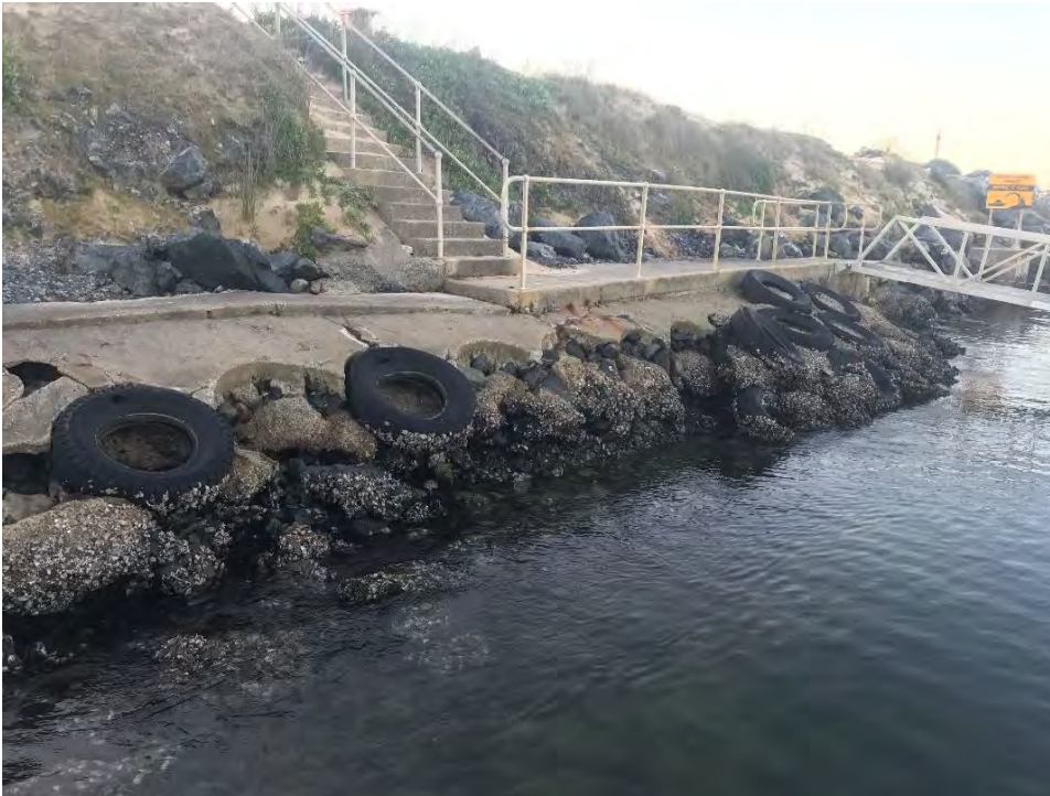
Figure 20: Existing concrete and tyre revetment in state of significant disrepair
