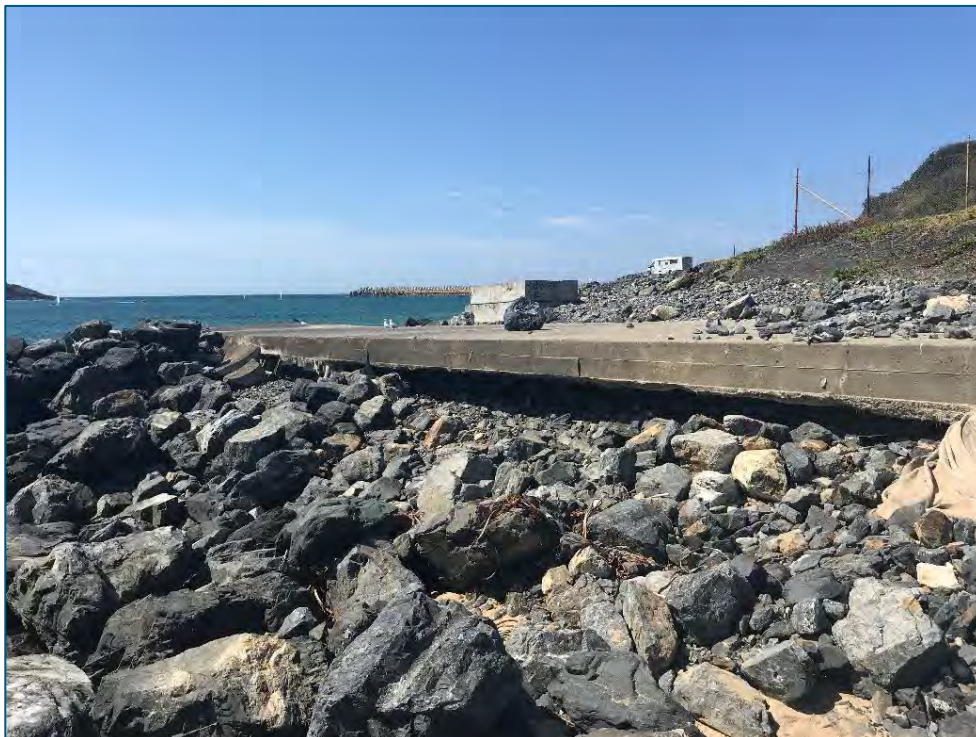
Figure 22: Damaged area adjacent to the existing Material Offloading Ramp
