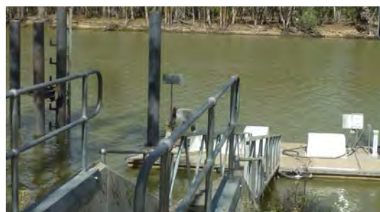
Dareton - Sewage Pump Out
