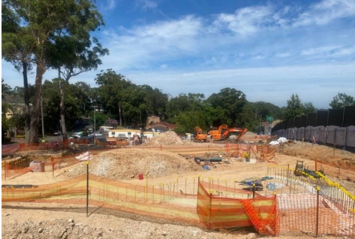
Construction work progressing at the North Rocks Commuter Car Park in February
