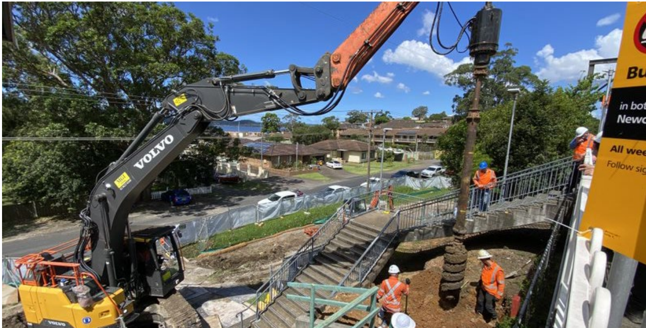
Piling work for the platform extension on the Kurrawa Avenue side of Point Clare Station, April 2022
