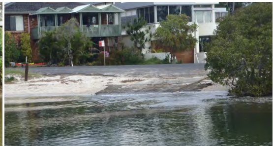
Winda Woppa boat ramp. Single lane does not meet demand. Poor surface conditions and no supporting facilities
