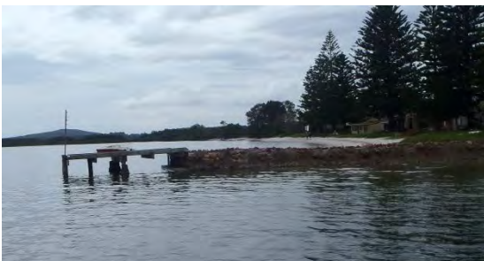
Poor condition of jetty at Taylor's beach. Pontoon extension for low water levels and upgrade of structure required
