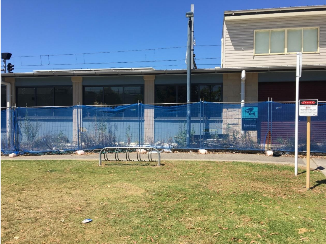
Figure 1-6 The existing bicycle rack at Revesby Station, proposed to be replaced, looking south
