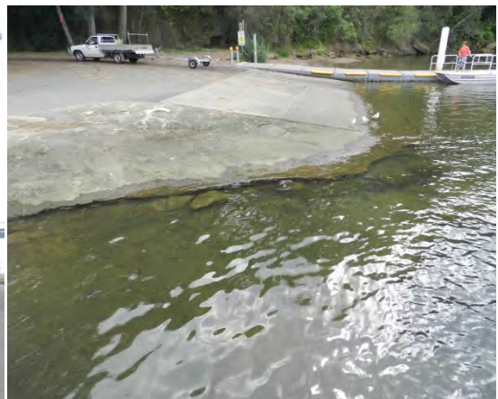
Greys Beach boat ramp. Opportunity to widen ramp and provide more lanes to meet demand
