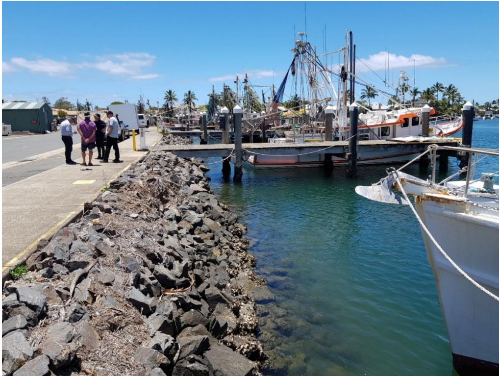
Figure 16: Existing rock revetment and berthing zone to the east of the proposed works
