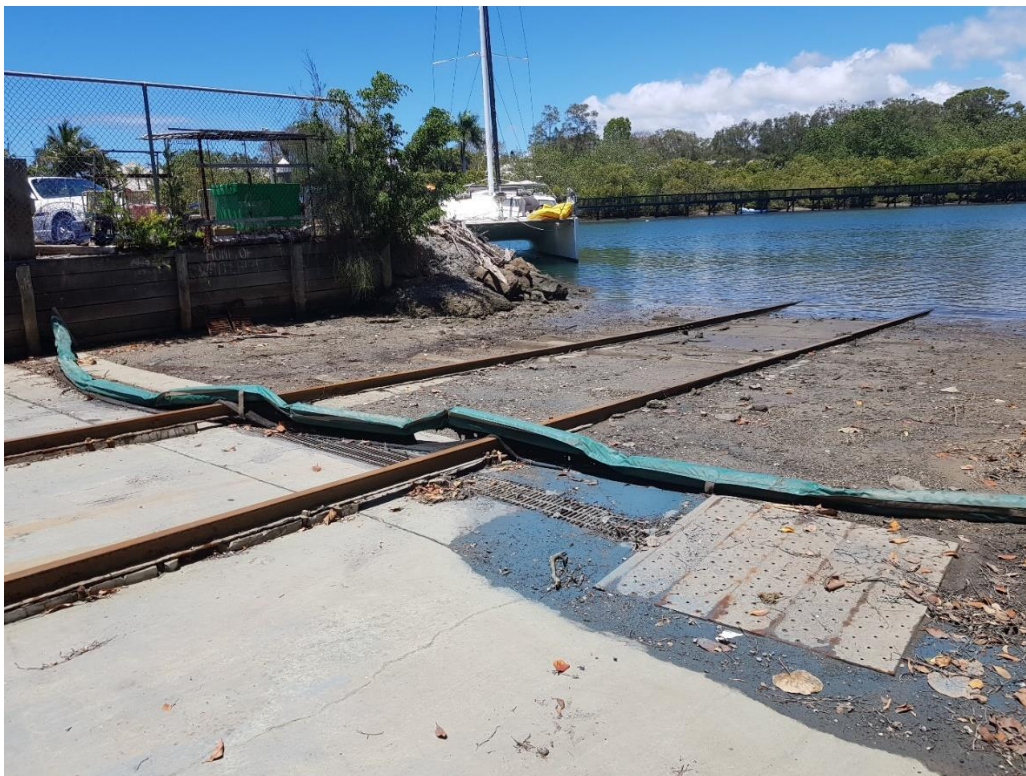
Figure 13: Image facing south down the existing boat ramp with the drainage grate/pit visible below the highwater mark
