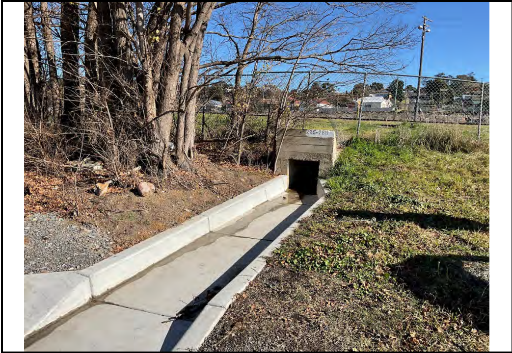
Photo 33: New drain installed on the east end of Ottiwell Street at sample location XS073. Drain appears to run under the train line with no visible starting point, potentially coming from the site.
