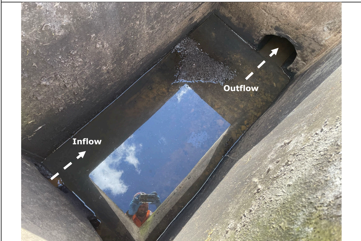
Photograph 26 Standing water sampled at SW02. Note the slight sheen on the surface of the water
