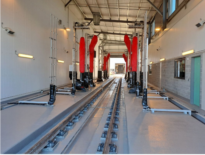
Train wash facility
