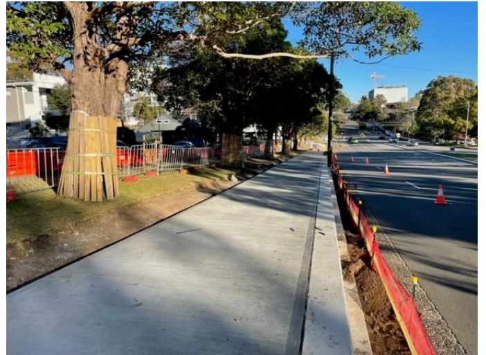
Above: Images of active transport link construction near Miranda Road and Jackson Avenue, July 2023
