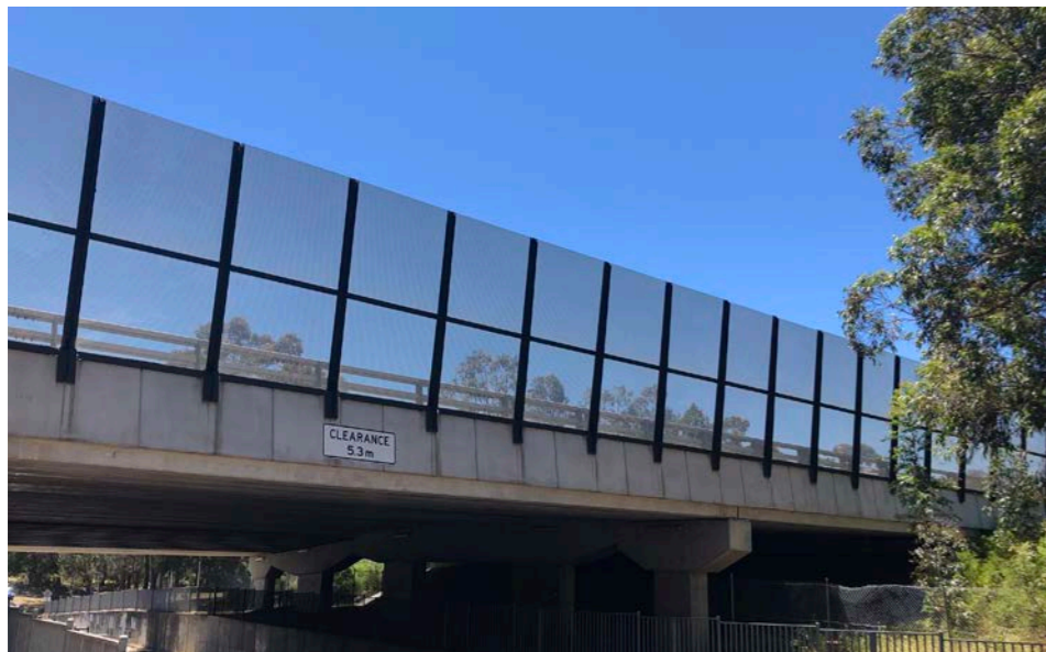
Figure 80: Example image of Throw Screen Type 1 - Penshurst Road Overbridge, M5 East (Sydney)
