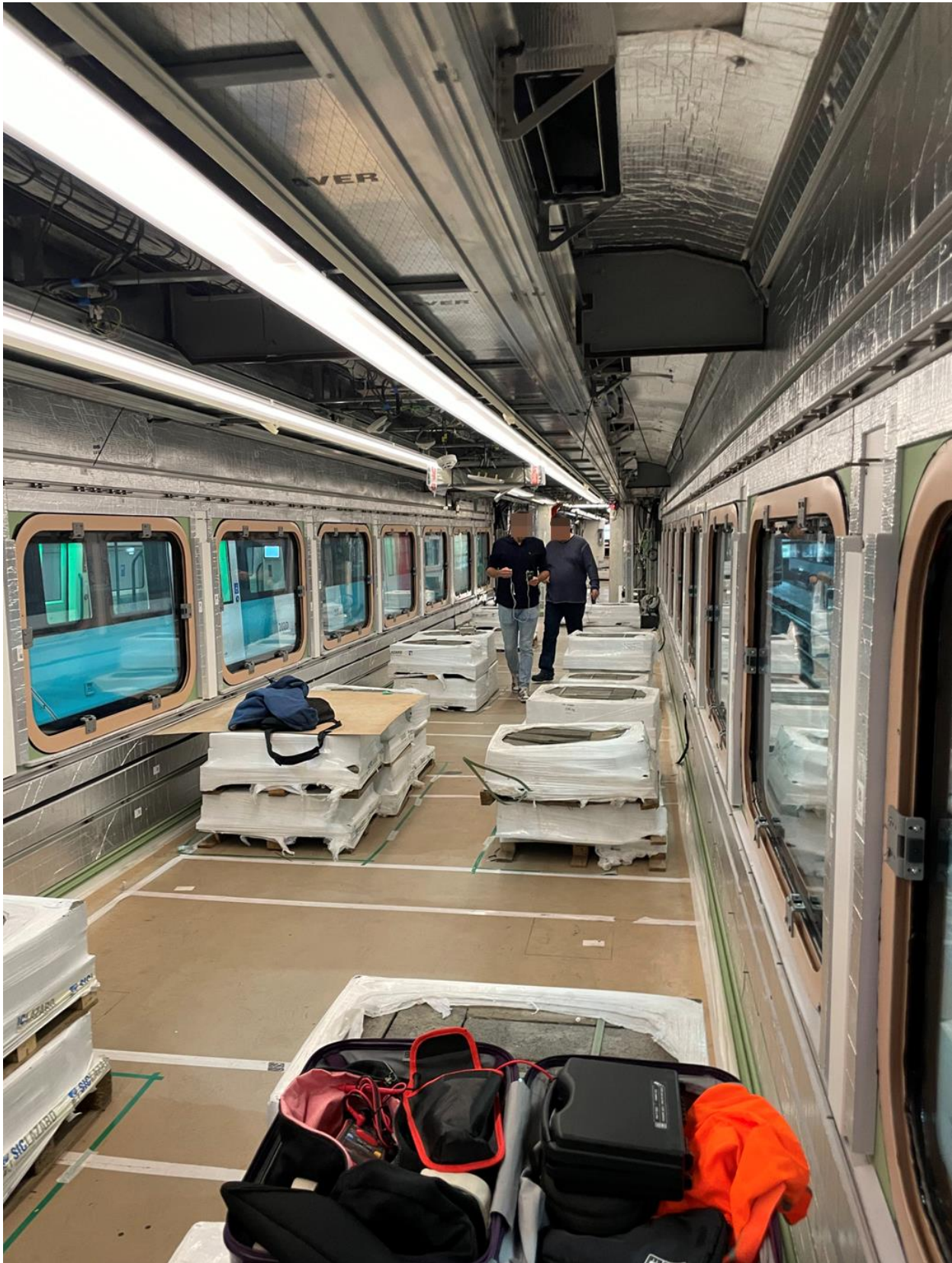
TfNSW and CAF reviewing the hearing loop installation on LR01
