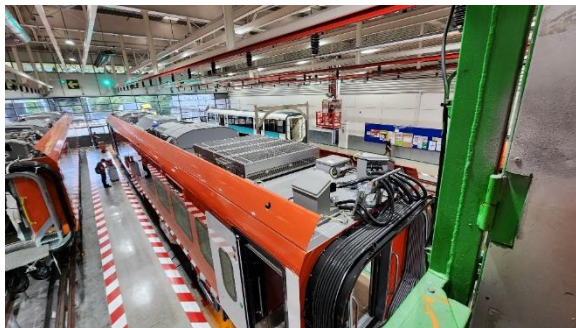
Roof mounted equipment
