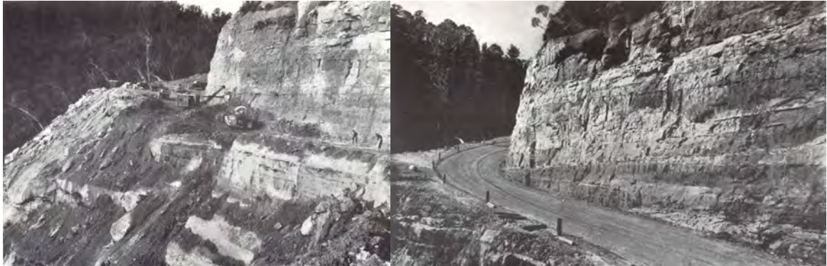
Figure 6-19: Mount Tomah road cutting under construction in 1947 (left) and completed in 1950 (right)
