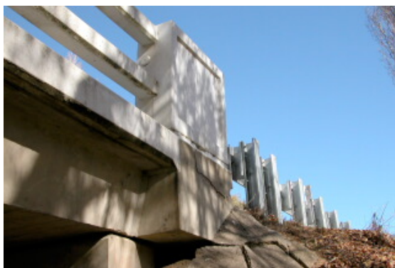
Endpost damage – Spring Creek (RTA Bridge No 1002) Bathurst
