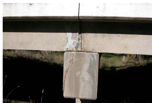
Spring Creek Bathurst (RTA Bridge No 1002) showing headstock and slab distress
