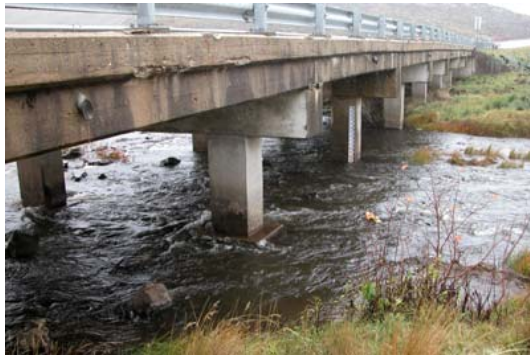
Bridge over Eucumbene River (No 6049) Freeze/thaw damage to kerb
