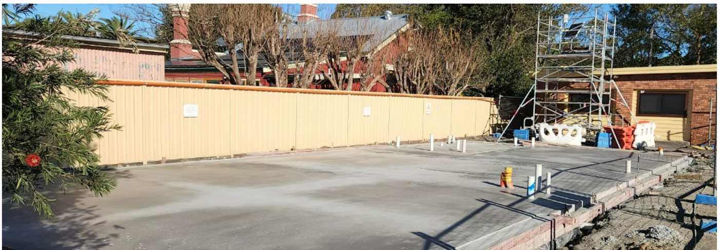
Concrete slab foundation work being completed at the location of the old maintenance centre, in preparation for the new one
