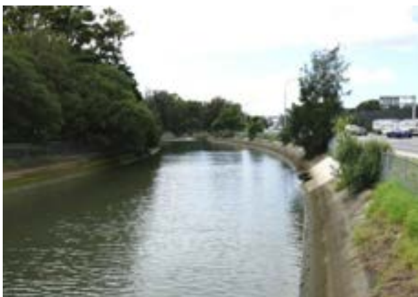
Figure 32 View to east along Iron Cove Creek Canal with Dobroyd Parade on the right
