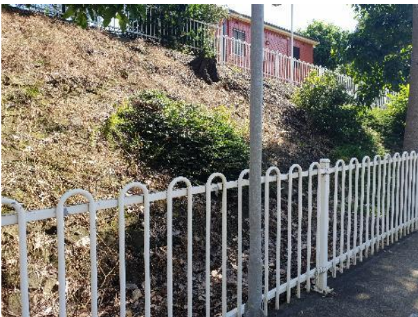
Photo 24 North-west-facing view of the overgrown stone retaining wall on the western side of the station
