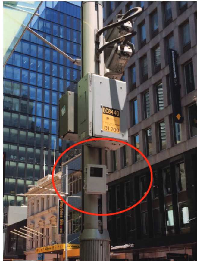
An example of a camera used for data capture mounted on a light pole
