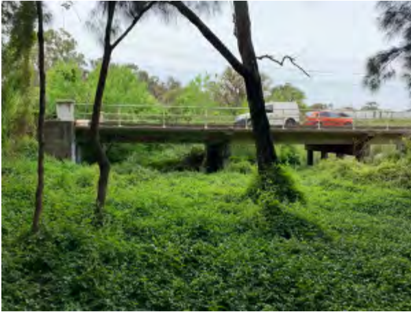
Photo 3.35 Aquatic Site 11 - The unnamed second order stream at the Auld Avenue bridge showing riparian zone
