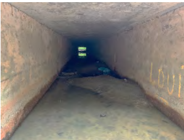
Photo 3.39 Aquatic Site 5 - Inside the culvert under Milperra Road showing the unnamed first order stream which drains south to the Milperra Drain
