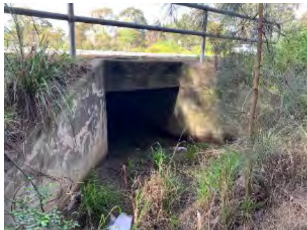
Photo 3.38 Aquatic Site 5 - The unnamed stream and culvert on the northern side of Milperra Road
