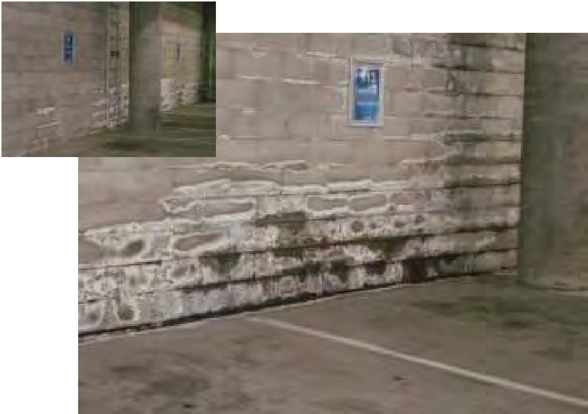
Parramatta/Georges River HGL – evidence of salinity in structure of Telstra Stadium, around the runway entrance to the stadium, Sydney Olympic Park. Salt crystals forming after evaporation of saline rising damp in brick work (Photo: DECCW/Charmaine Beckett).
