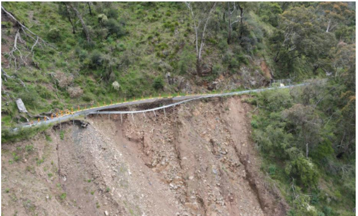
Figure 6-4 Viewpoint 2 –existing view from a drone at the main failure
