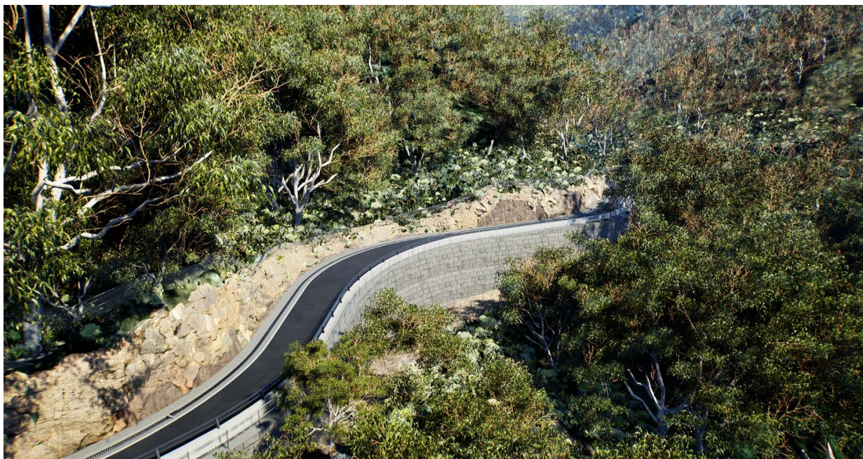
Figure 3-4 Reinforced soil wall – second failure
