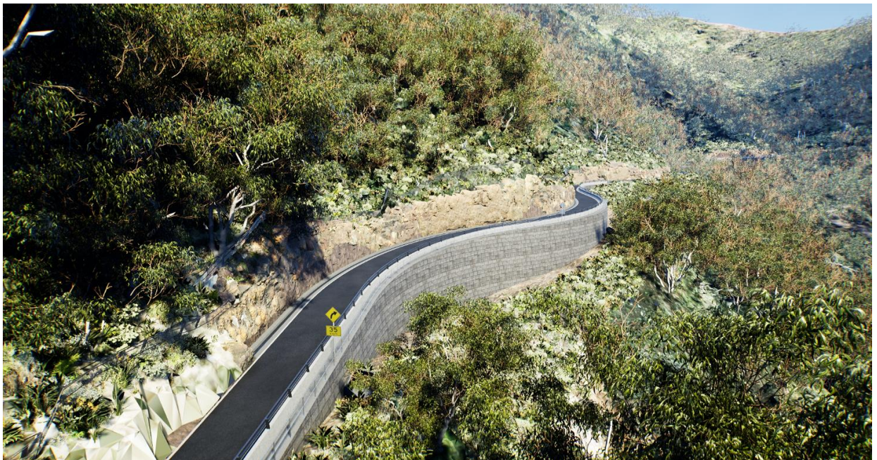
Figure 3-3 Reinforced soil wall – main failure
