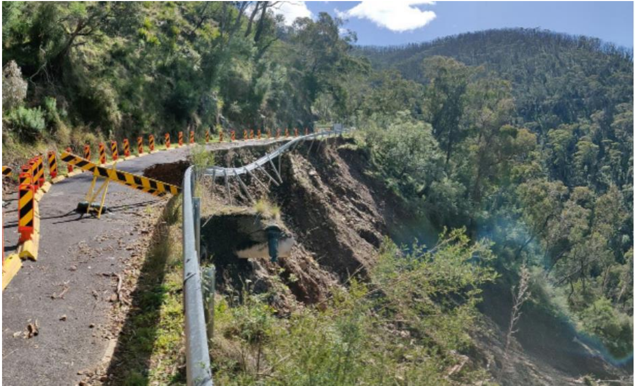
Figure 6-3 Viewpoint 1 –existing view from Jenolan Caves Road at the main failure
