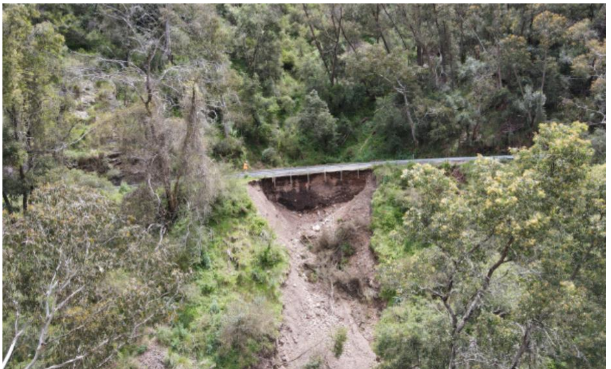
Figure 6-6 Viewpoint 4-existing view from a drone at the second failure
