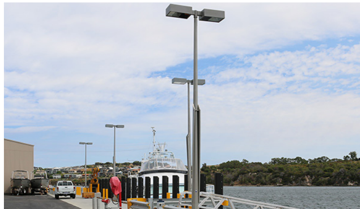
Tidal zone - Integrated higher level lighting
