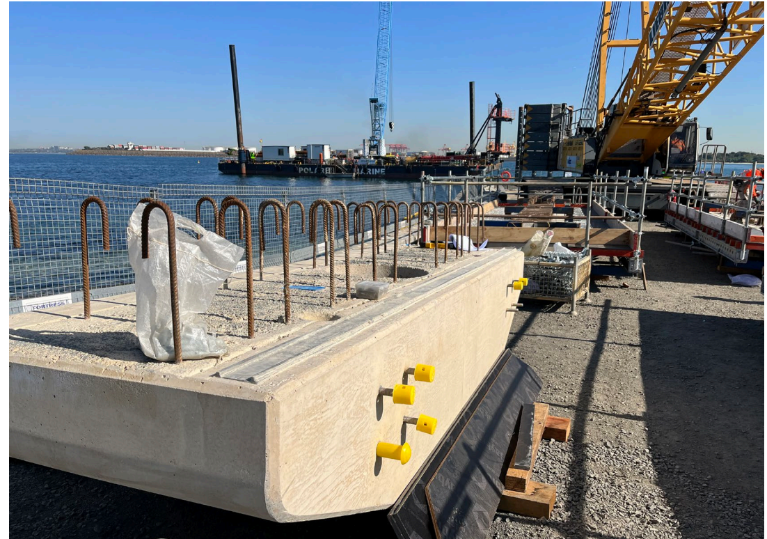
A pre cast wharf support beam (head stock)
