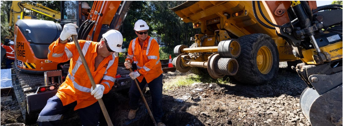
More Trains, More Services' construction team members at work in the rail corridor on the NSW South Coast in 2021
