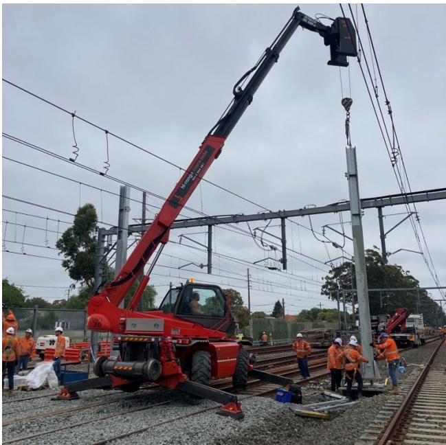
The project team installing infrastructure to support overhead wiring between Kingsgrove and Beverly Hills in 2022.
