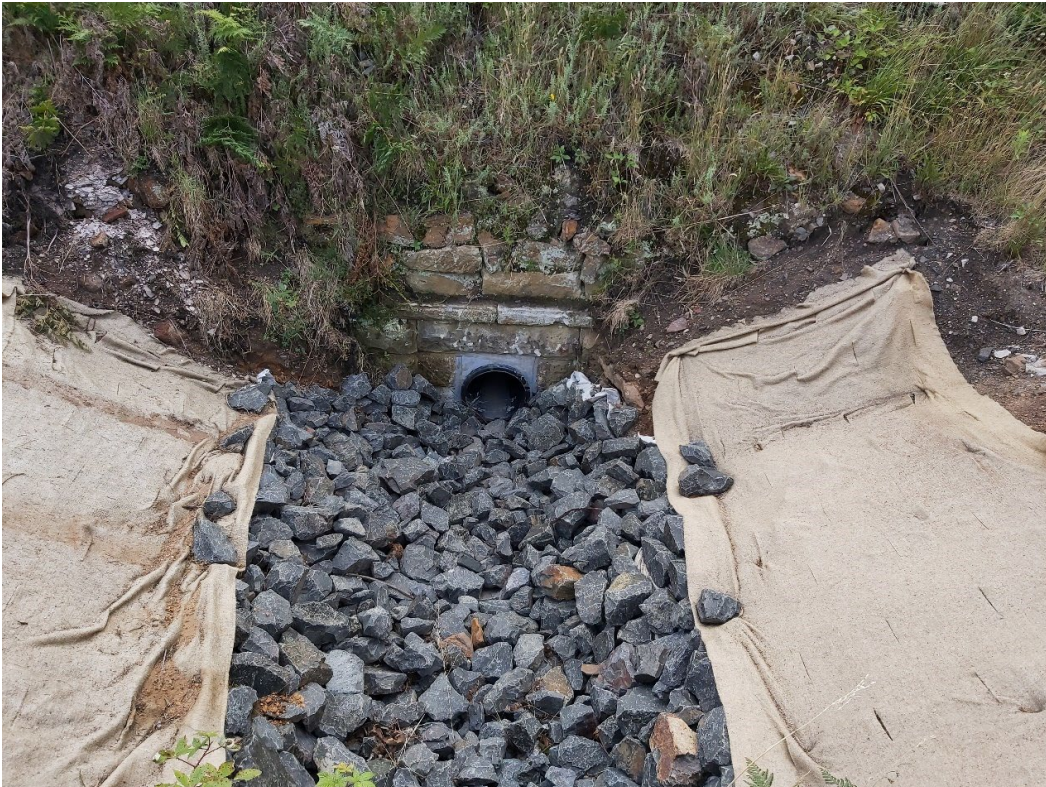
Figure 6-18: Sandstone culvert on western side of railway embankment, looking east (RPS, 2021b)
