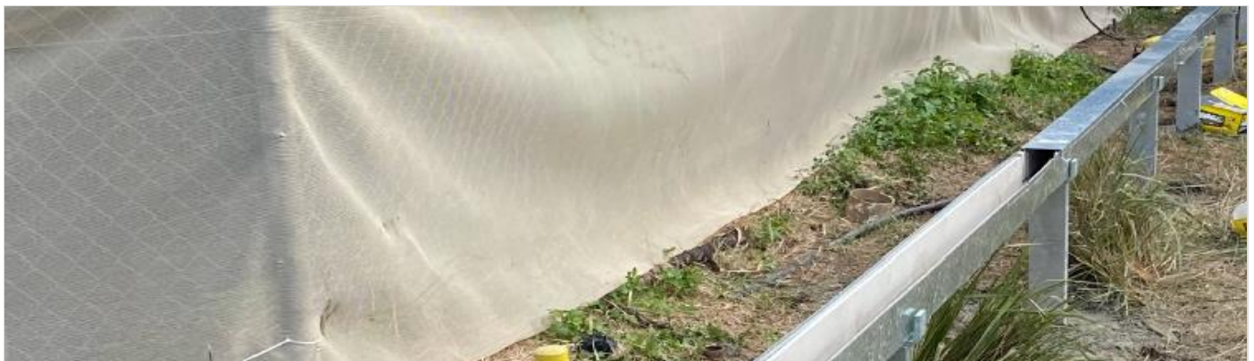
Galvanised steel trough installed on Burren Street near Macdonaldtown Stabling Yard in May. In July we will feed cables through the trough to support new signalling infrastructure inside the rail corridor.
