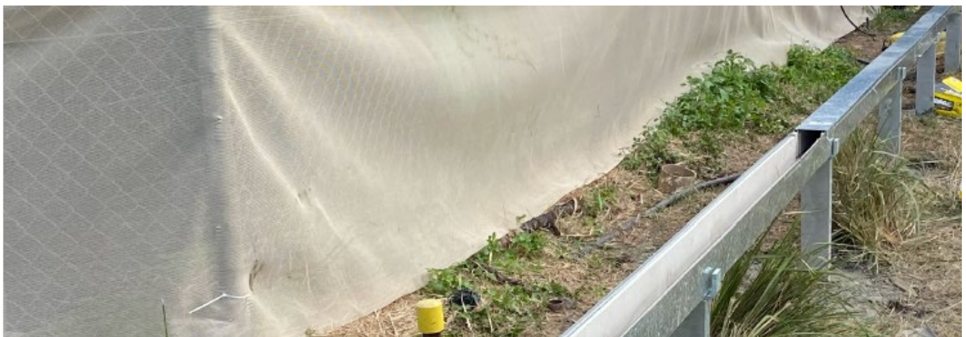
Work to install a new galvanised steel trough on Sydney Trains land at the end of Burren Street took place in May 2022. In the coming months we will feed cables through the trough to support new signalling infrastructure inside the rail corridor.
