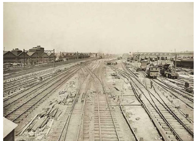
Photo taken during Illawarra Dives construction around 1926. The dives were constructed using one of the oldest methods of tunnelling known as 'cut and cover'. This method involves digging a trench, which is then covered by a concrete deck.
