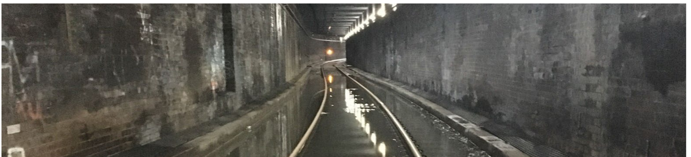
Drainage upgrade work will prevent future flooding inside train tunnels in Eveleigh
