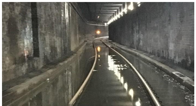
Flooding event in the Illawarra Dive tunnels at Eveleigh. Work is underway to improve the drainage system in the area and prevent future flooding in the rail corridor.
