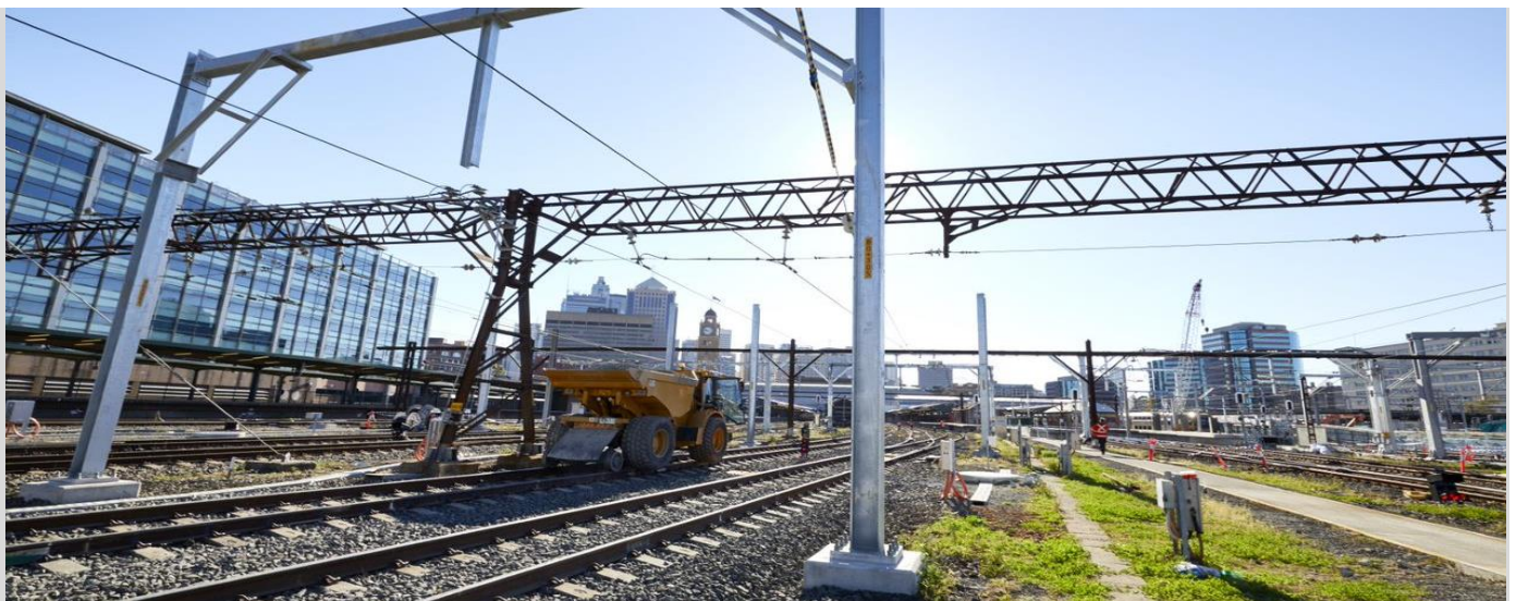
Work undertaken at Central in 2021 as part of the Sydney Terminal Area Reconfiguration Project
