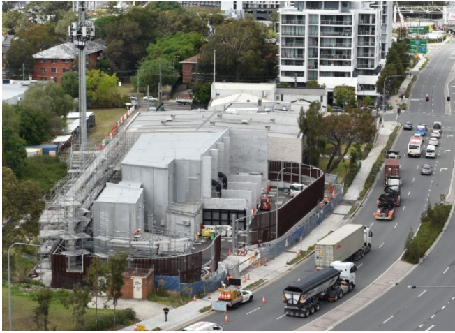
Progress photo of the fence installation taken in September 2023. The upper fence will reach 10.5 metres and installation will continue in November and December 2023.
