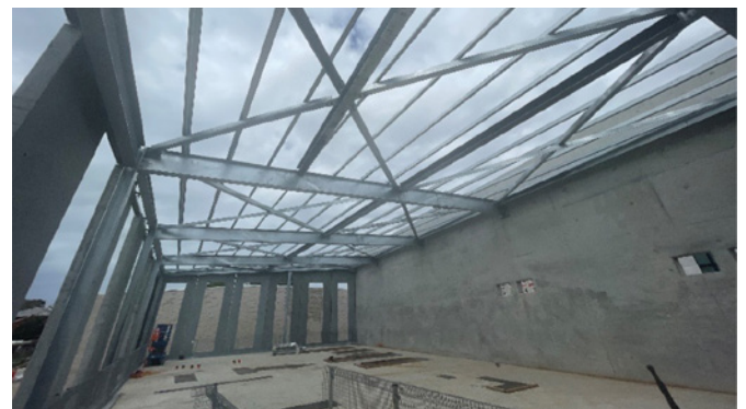
Progress on the southern building of the substation prior to the recent roof installation
