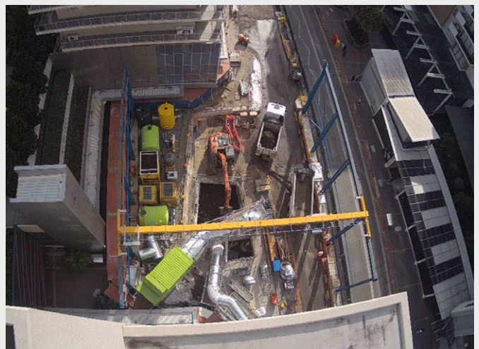
Aerial view of work on the new western station entry in July.
