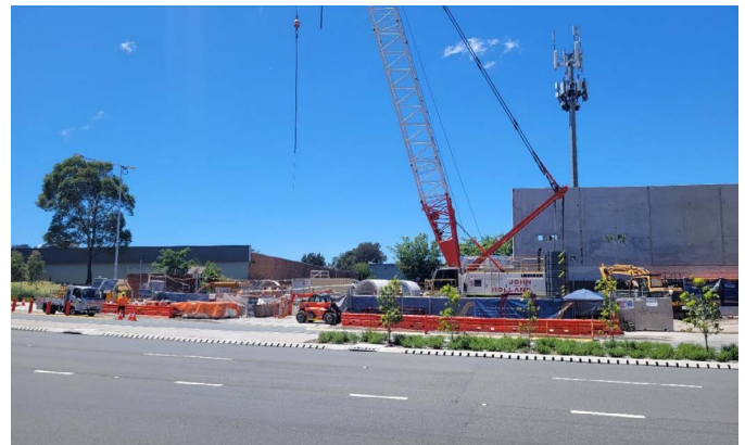
Work is progressing at the future substation site at 166 O'Riordan Street, Mascot.
