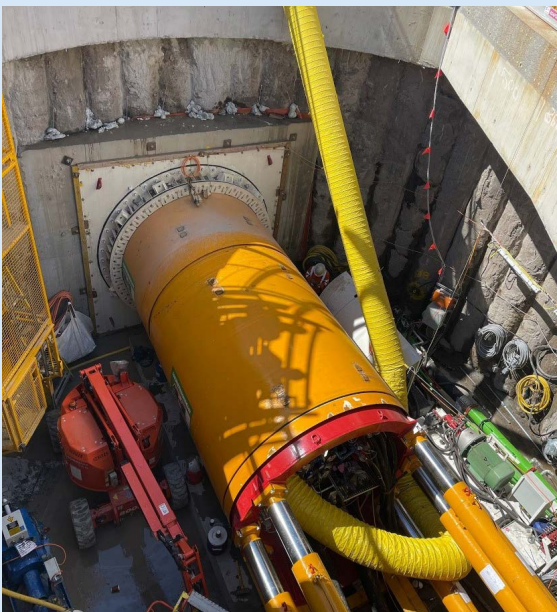
The micro tunnelling machine launch in early November from 200 O'Riordan Street, Mascot.
