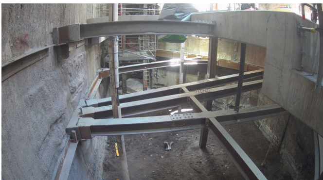
Digging to the concourse level at the site of the new western entrance of the station.
