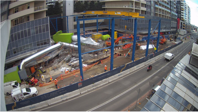
Work on the new western entry setting up the ventilation and dewatering plant and equipment within the site compound.
