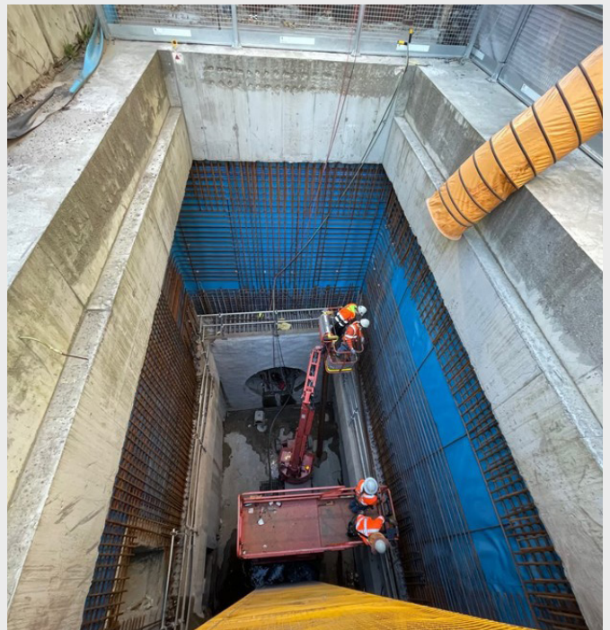
Steel fixing at the retrieval shaft on Bourke Street between Coward and John streets.
