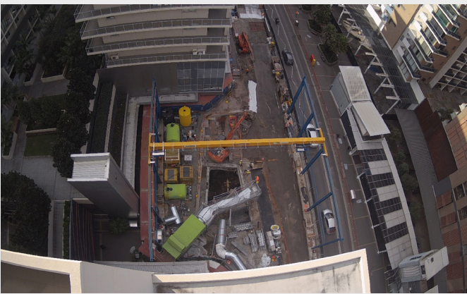
View of the Mascot Station Access upgrade work showing progress during June.
