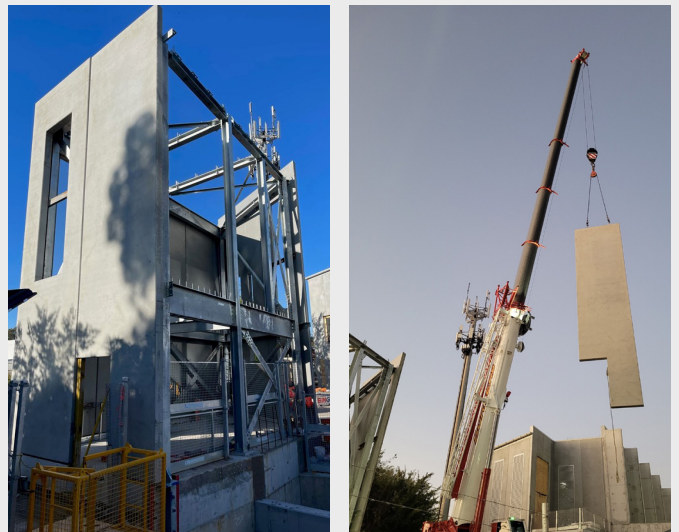
Northern section of the substation building taking shape following the installation of precast panels.
