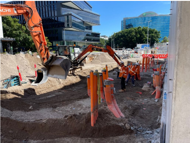
Excavation in preparation for the installation of the transformers at the future substation site.
