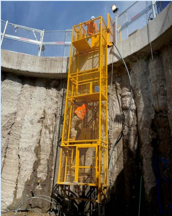
View from inside the launch shaft for the micro tunnelling machine at 166 O'Riordan Street.
