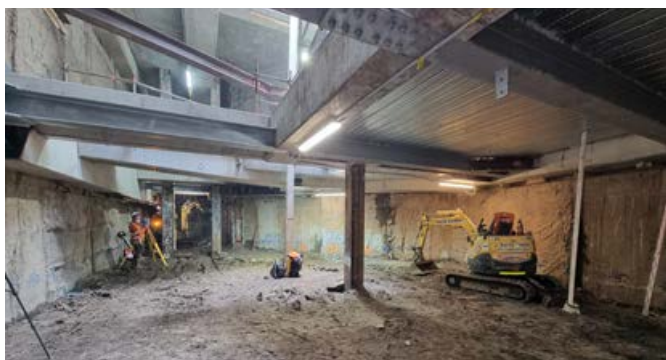
Excavation to the underside of the temporary propping level for the new western entrance of the station on Bourke Street.
