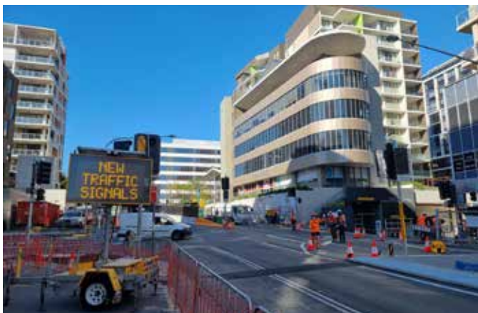
Preparing for the new temporary traffic signals at the corner of Bourke and John Streets
