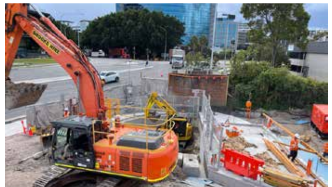
Excavation of the launch shaft at 166 O’Riordan in preparation for the tunnelling this month.
