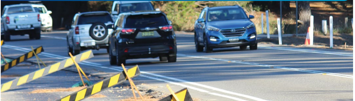
Noise and vibration mitigation measures will be used to minimise impacts during construction
